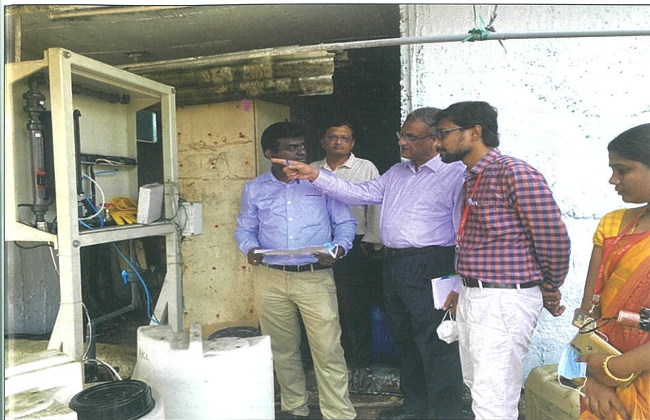
Pilot unit for demonstration of application of ClO 2 for improving process water quality and odour control.
